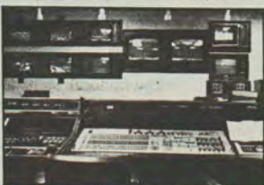
The House TV control room
